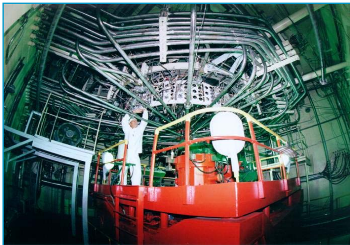
Reactor View from Reloading Machine Side
