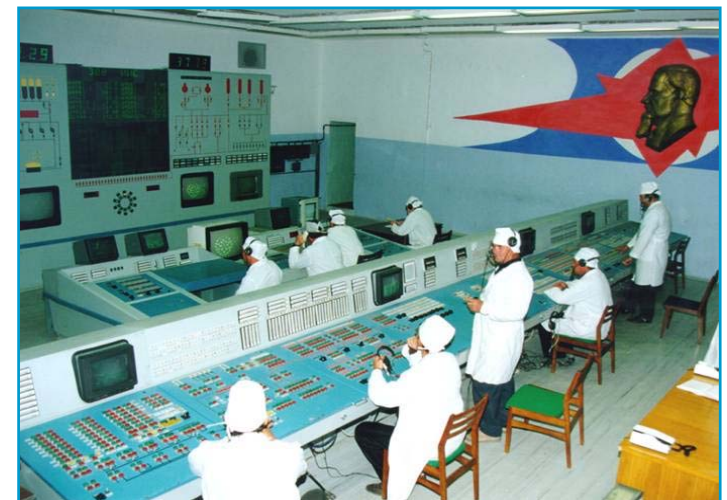
Reactor Control Room
