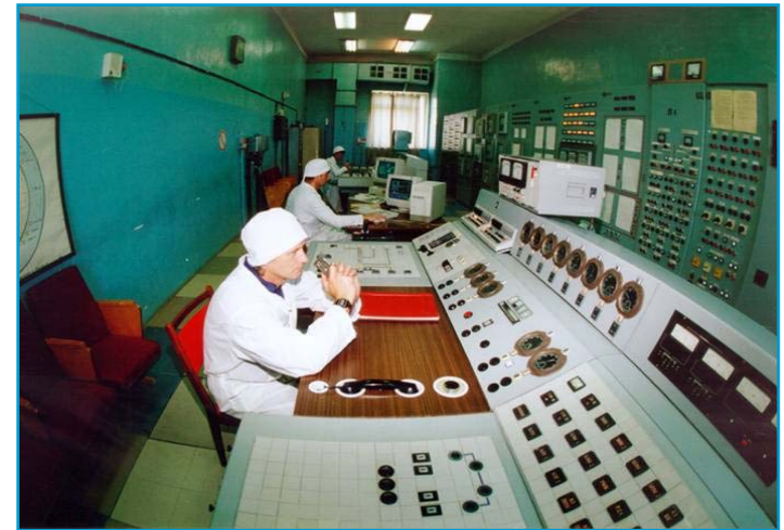
Reactor Control Room
